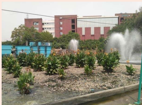
ETP Laundry Unit
